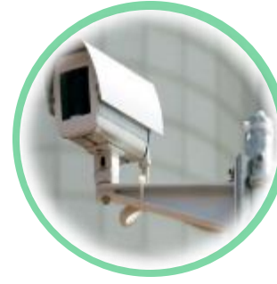
CCTV and street lighting with smart poles and LED lights.
